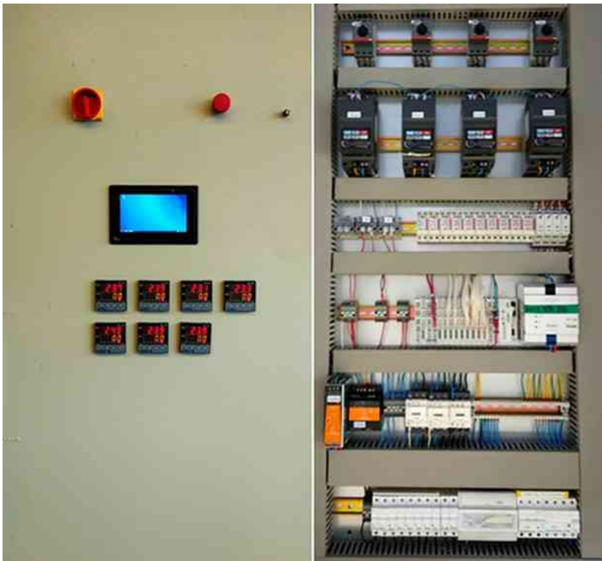
Figure 3-20. Programmable logic controller
