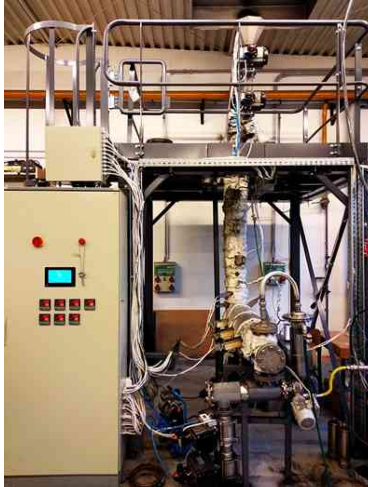
Figure 3-10. Multi-stage gasification system at the University of Miskolc, Hungary
