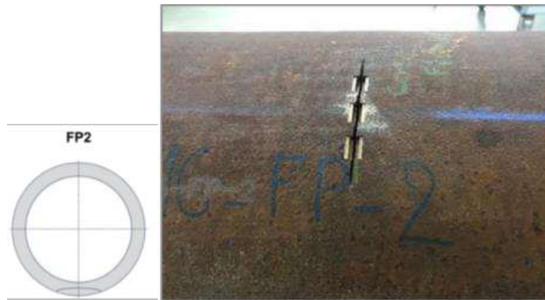
Figure 57 initial crack defect FP2
